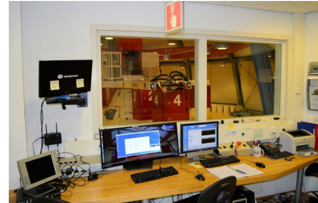
LDC control room
